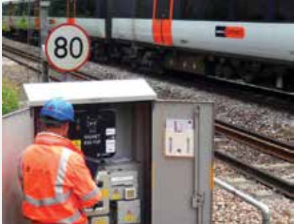
Camlin designs, manufactures and provides solutions to the global energy and transport sectors
